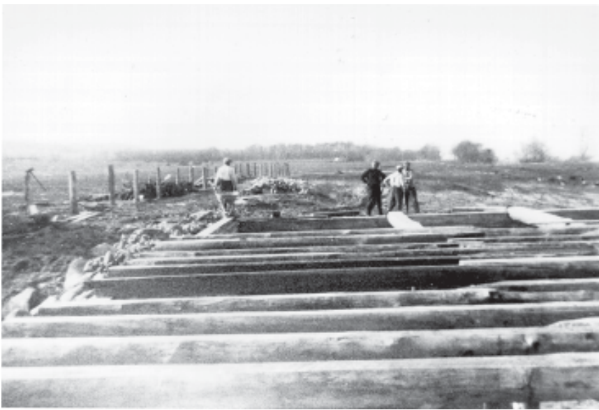
Figure 4.5. Manitou Island Association barn during construction, 1927. The large, modern, gambrel-roofed barn was the centerpiece of the MIA's farmstead at North Manitou Village. It was built on a site amidst the farm formerly operated by Silas Boardman and the Newhalls.
