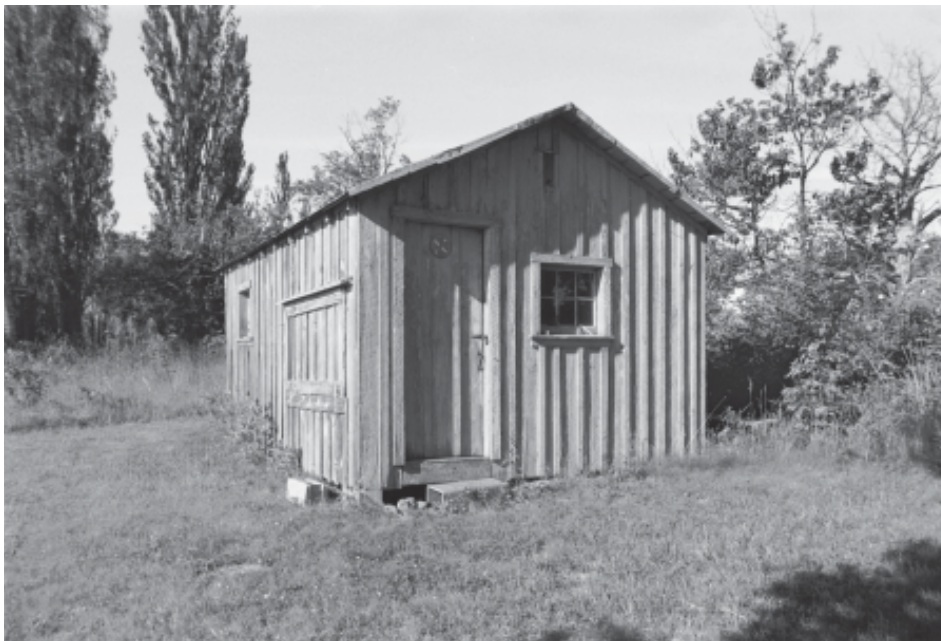
Figure 4.127. Migrant orchard workers' cabin, 1996. The design of this former orchard workers' cabin, which is located behind the Alford cottages, is nearly identical to that of the three structures standing north of the village. This cabin, however, is in superior physical condition.
